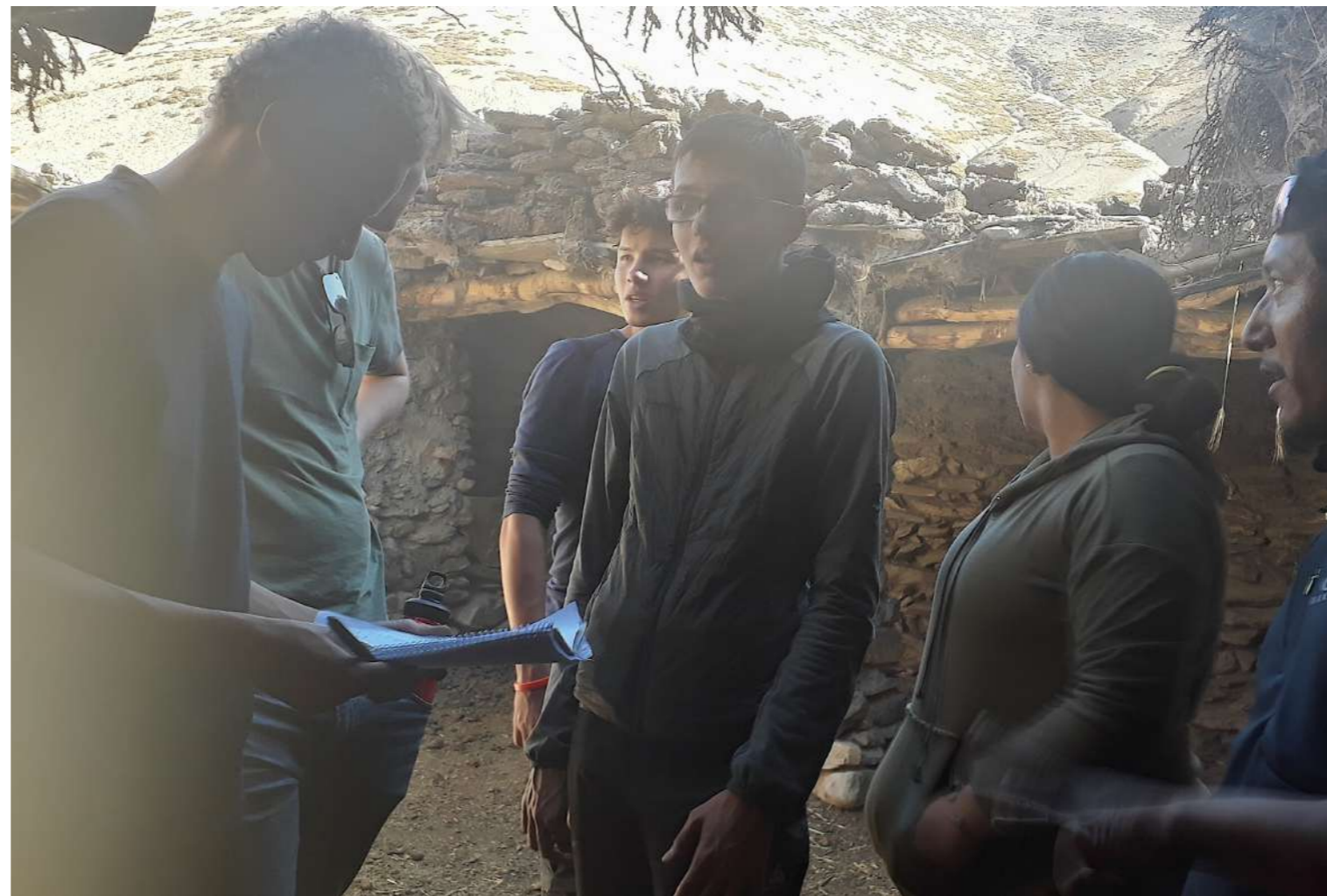
Electrification begins. -Stanzin attaches a bulb holder inside one of the homes. -The students of ISZL discuss the location of the holders. Stanzin helps them in this to plan the optimum approach so that we don't lose time.
